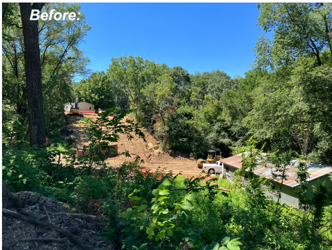
A view of the construction site, Summer 2022, with the sewage treatment plant at the lower right.
