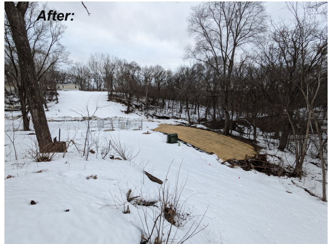
View of the construction area after the project wrapped up, leaving a large, flat area near the river waiting for the community's next plan.
