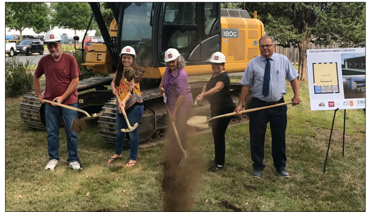
Park Plaza Board Members (pictured above) at the groundbreaking of their new stormshelter in August 2018.
